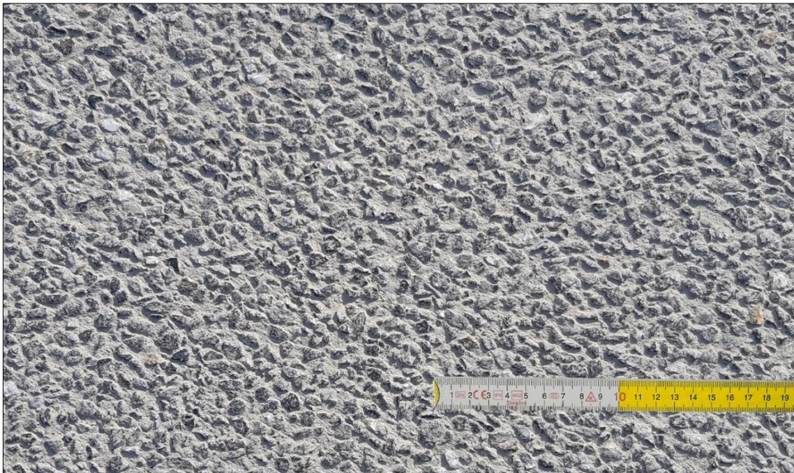
Figure 14. EACC road surface
